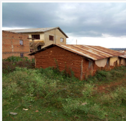
Figure 10a: New & Dilapidating Houses in Kitere.
